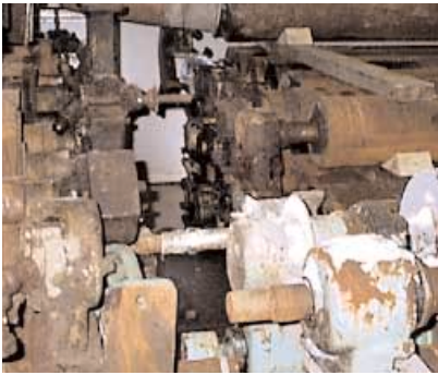
Felt rolls prior to reconditioning.
