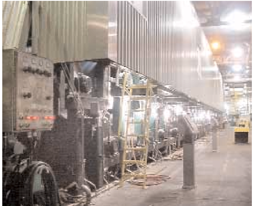
Tending side of the dryer section.
