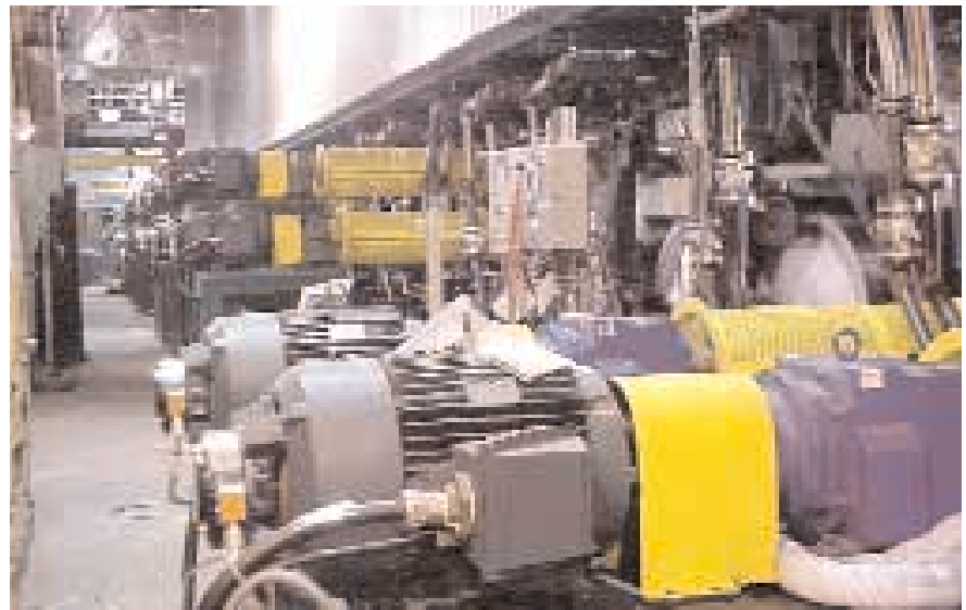
Drive side of the dryer section.
