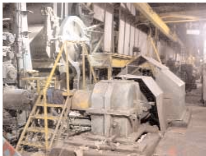
Original line shaft drive.
