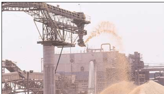
The new woodyard delivers over 99.3% accepts to the Interstate board mill—at over double the per-hour production rate of the previous woodlot installation.
